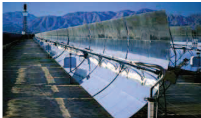
Solar-thermal parabolic trough power plant
